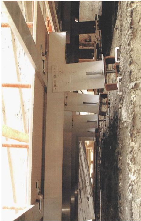
Image-No. 9 Dubai – complicated, error prone distance bridging construction, assembled with standard aluminum sub-constructions. –Are these structurally safe?
