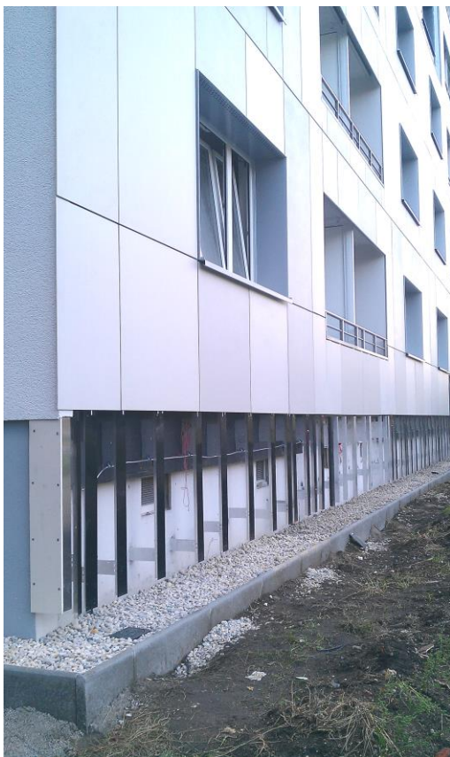
Image-No. 7 An aluminum wall fixing done on a at the time standard facade (Estate in Dresden)
